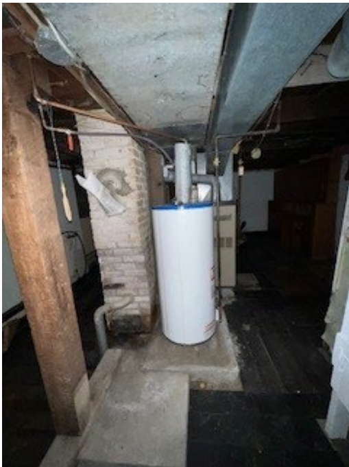
Basement / Water Heater
