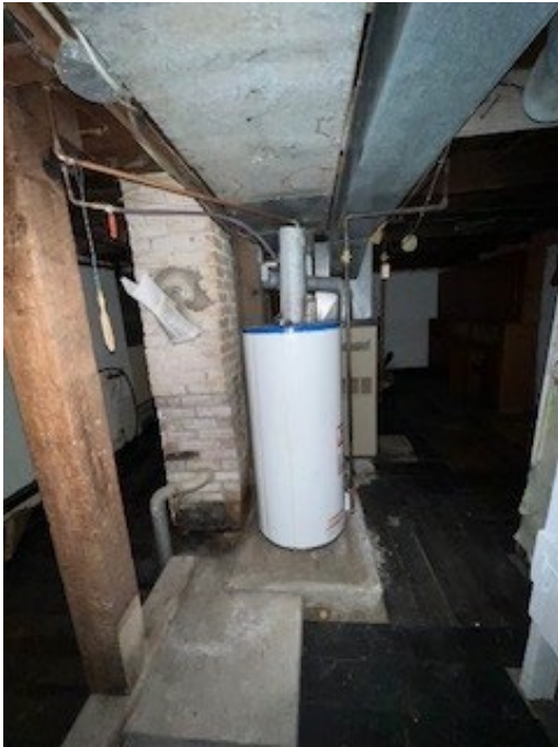
Basement / Water Heater
